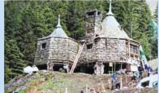
Construction of 'Hagrid's Hut' in Scotland for Harry Potter and the Prisoner of Azkaban.
